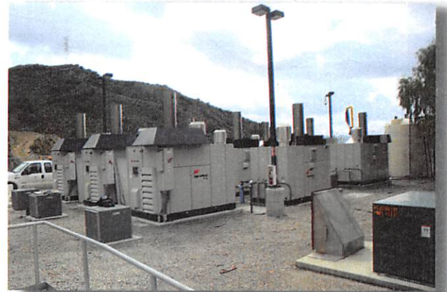
Microturbine Electrical Generation Facility
